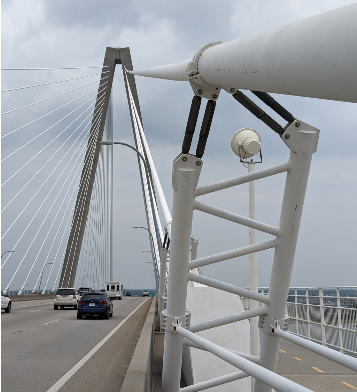
The Arthur Ravenel Jr. Bridge spans the Cooper River outside of Charleston South Carolina (USA) with a main span of 471 m (1,546 feet) and uses dampers on the center cables to mitigate wind and traffic-induced vibrations in the structure. It is the third longest among cable-stayed bridges in the Western Hemisphere (2023).
