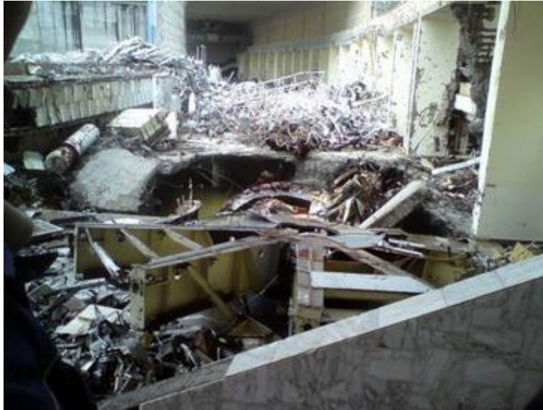
Figure 2.28: Sayano Shushenskaya's turbine hall after the accident b .
