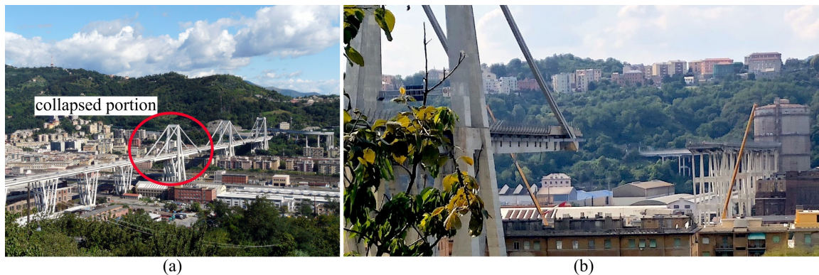
Figure 7.1: The Ponte Morandi bridge, showing the bridge: a) before the collapse b , and; b) after collapse c .
